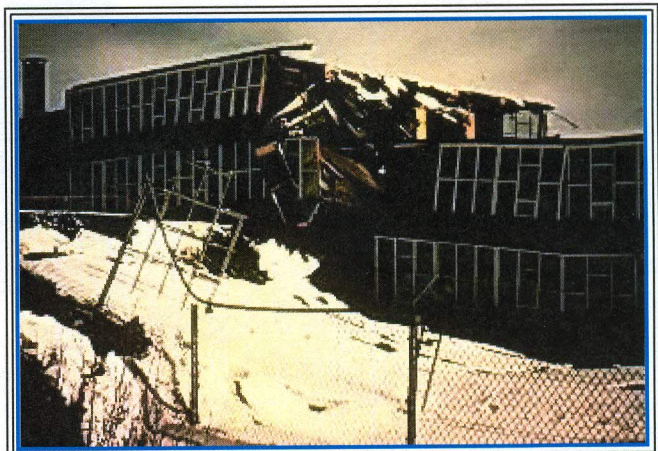
This photo shows evidence of the subsidence at the Government Hill School location, Anchorage.
